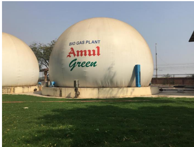
Fig. No. 4.2. BIOGAS PLANT
